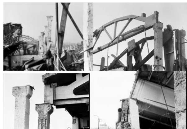
Figure 1. Types of destroyed one-storey frame buildings due to the destruction of the nodes of connection of rafters with columns in Leninakan city (now - Gyumri city)
