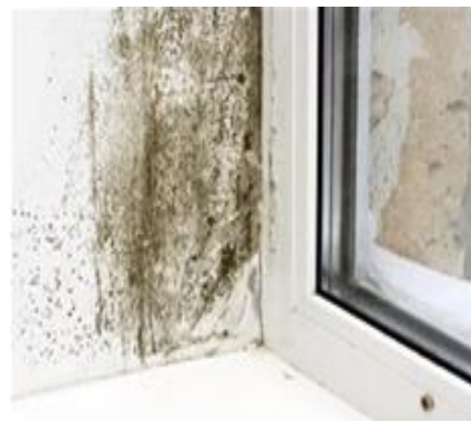
Figure 22. Mold or black spots in wall to be cleaned by Javel water
