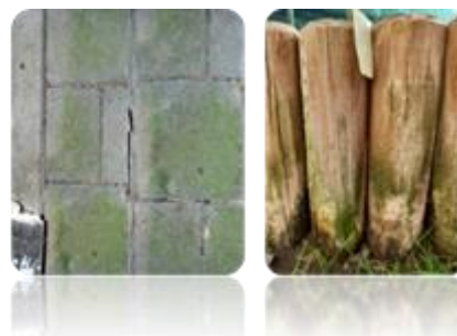
Figure 1. An example of the occurrence of biological corrosion on serviceable surfaces
