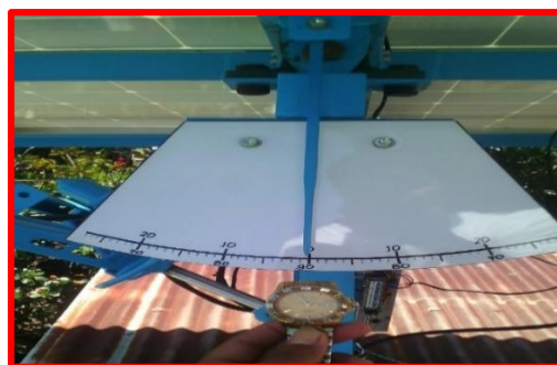
Figure 25. Alignment of the PV module during Noon-Sun Angle @ 1PM on February 07, 2023
