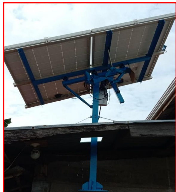
Figure 18. Actual Picture of the Single Axis Solar Tracker System
