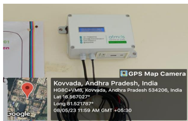
Figure 1. Shows the Atmos particulate matter sensor installed inside a room of the Engineering College Campus, Bhimavaram, India
