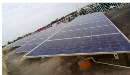
Figure 1. Picture depicts 100 KWp power plant established atop VIT Block, Bhimavaram, India
