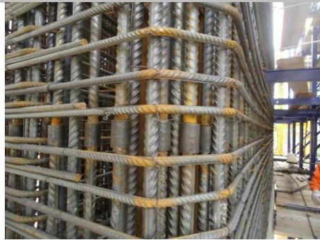
Figure 25. Couplers type A in the pier P3
