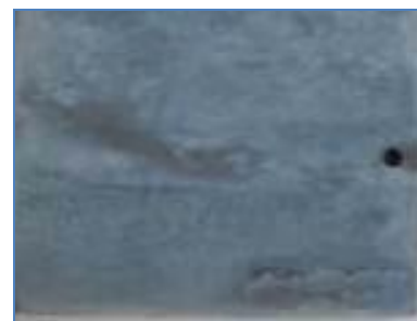
Figure 6. The appearance of the coating after the corrosion resistance tests
